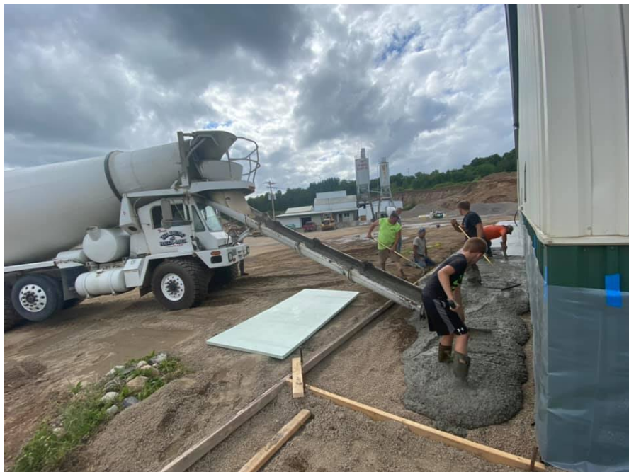
The concrete being poured in this photo is derived from aggregates. Source: Tony’s Wabeno Redi-Mix, LLC, 2020.
