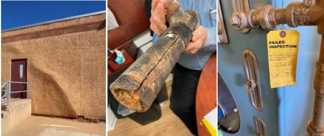
From left to right: A crumbling foundation at Many Farms Community School (work orders submitted July 10, 2008); a corroded water line pipe at To'Hajiilee Community School (work orders submitted September 20, 2021); and an inoperable boiler that failed inspection at Many Farms High School (work order submitted January 9, 2008). 15
